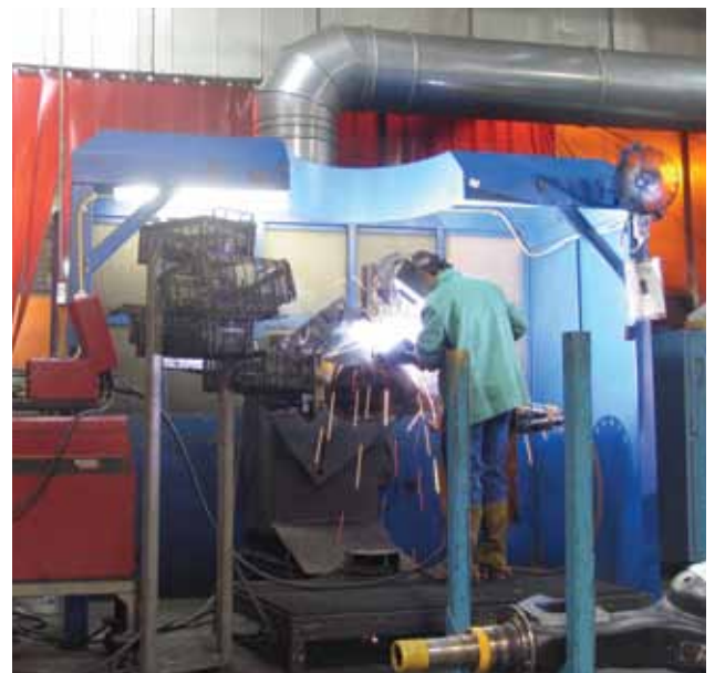
RoboVent CrossFlow System for a Manual Welding Process.
