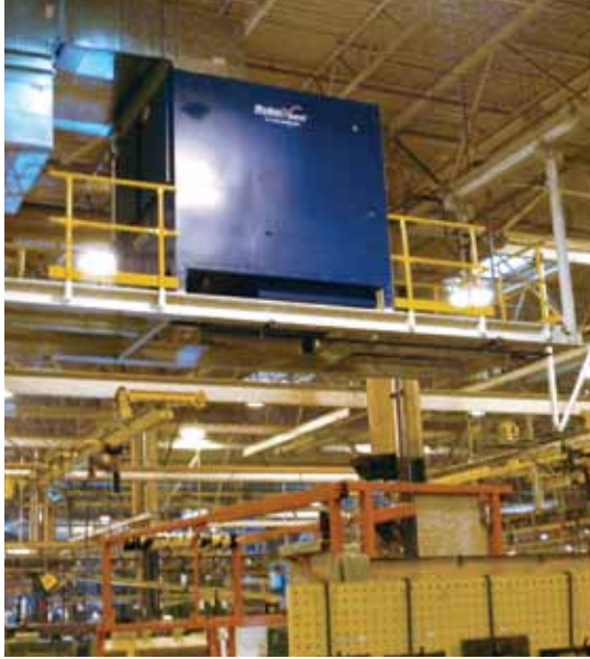
Ceiling-Hung RoboVent System with Mezzanine.
