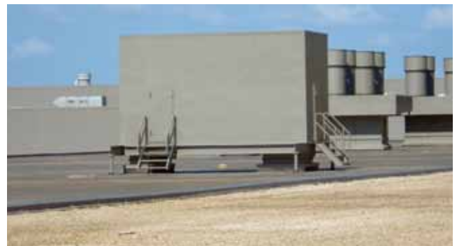
Roof-Mount RoboVent System in Enclosure.
