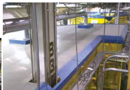
RoboVent Flexan Hood encloses a large Resistance Welding process.
