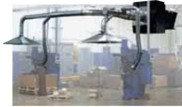
Ducted to each station
